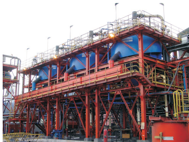
FIG 8 - The Imhoflot flotation plant at Huasco.
