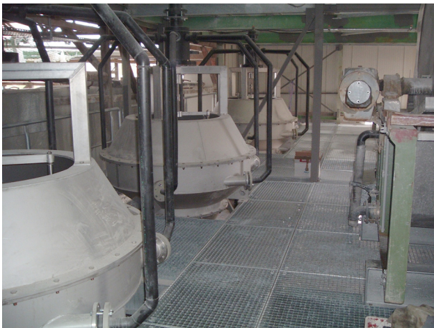
Figure 7: Dorfner flotation plant installed
